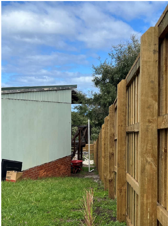
Figure 1: Photograph taken on the 10 October 2023 from the verge of the subject property showing the retrospective stair case in relation to the northern lot boundary.
