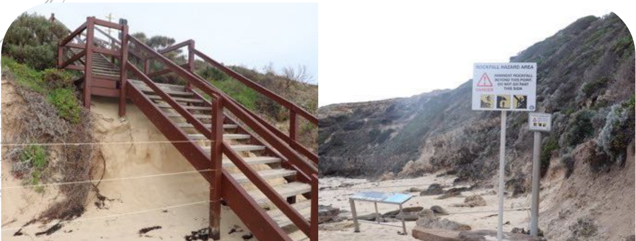
Figure 2.5 - Erosion under beach access stair near Surfers Point (left), and coastal rockfall signage and fencing at the base of the Riflebutts cliffs (right).
