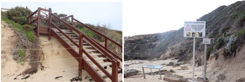
Figure 4-4 Erosion under beach access stair near Surfers Point (left), and coastal rockfall signage and fencing at the base of the Riflebutts cliffs (right).
