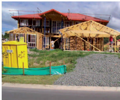
Sediment control fence along the lower edge of a residential building site
