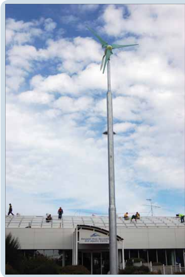
The 1 kw wind turbine (Zephyr) is the first of its type to be installed in the Southern hemisphere
