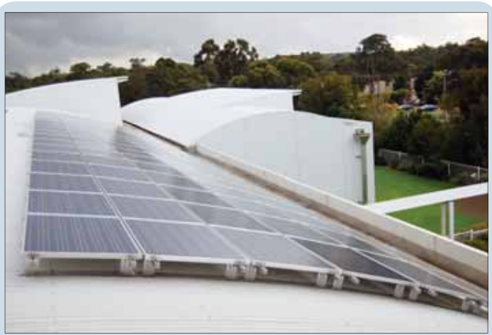
Solar Panels installed on the Recreation Centre roof.
